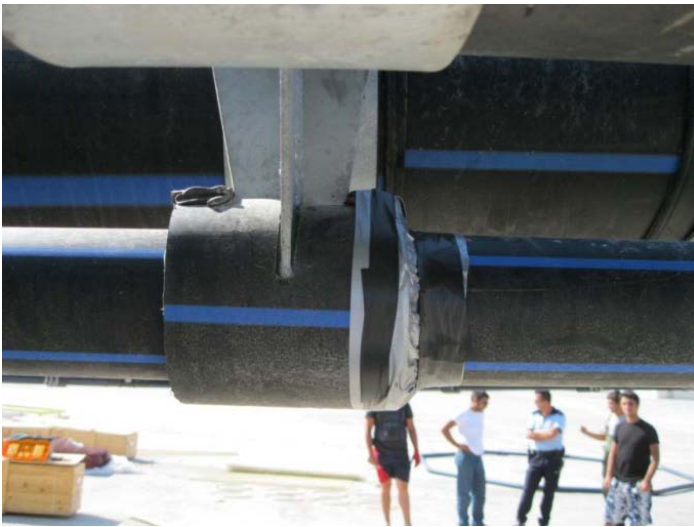
Figure 13. Insulating tape covering exposed metal to prevent galvanic corrosion.
